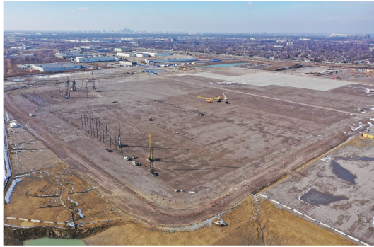
Once an empty plot of land, the 226-acre development now features two main buildings.
