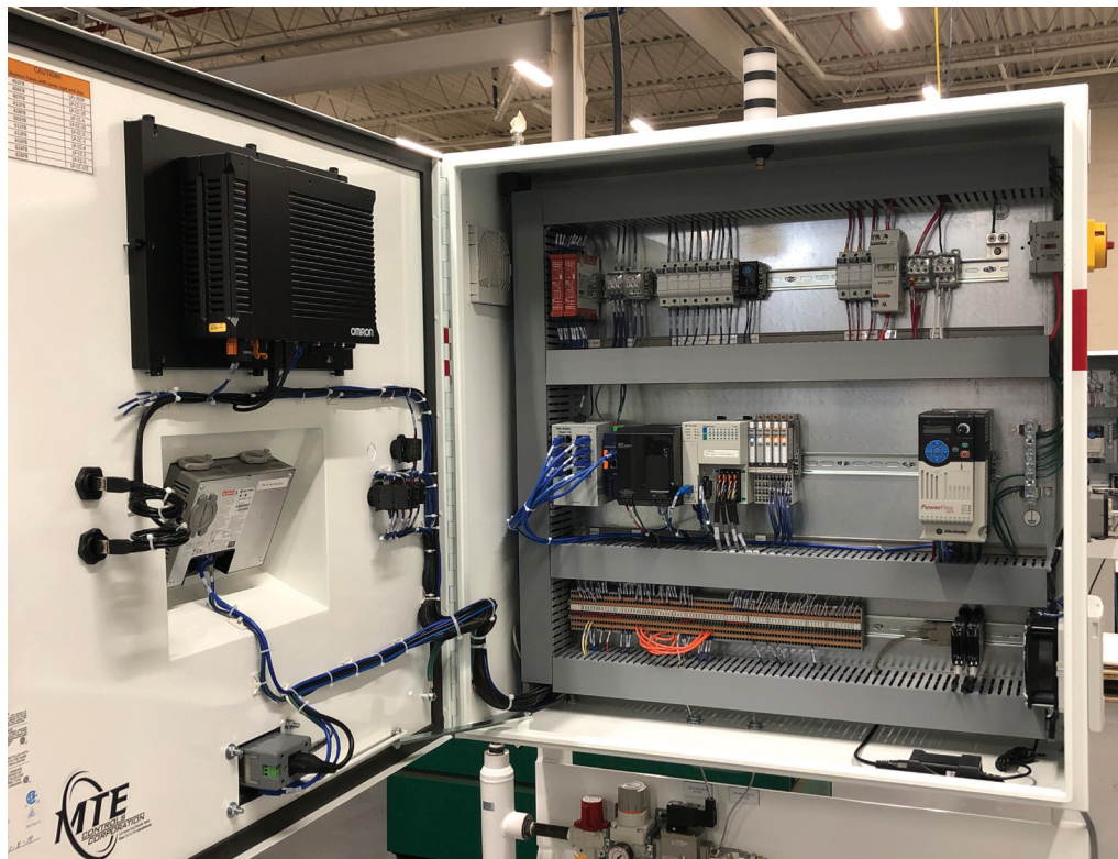
An example of control panels designed, built, programmed, and commissioned, in the MTE / Con-Syst-Int shop.
