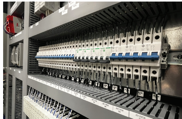
Servicing of a large industrial control panel for an interior parts bonding project in the automotive industry nearing completion.
