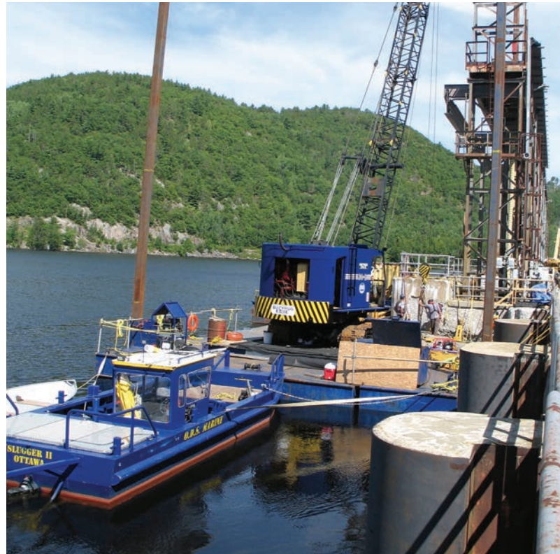
Seen here working on the Otto Holden Generating Station's coffer dams, ODS Marine's barge systems are able to meet any marine project's unique demands.
