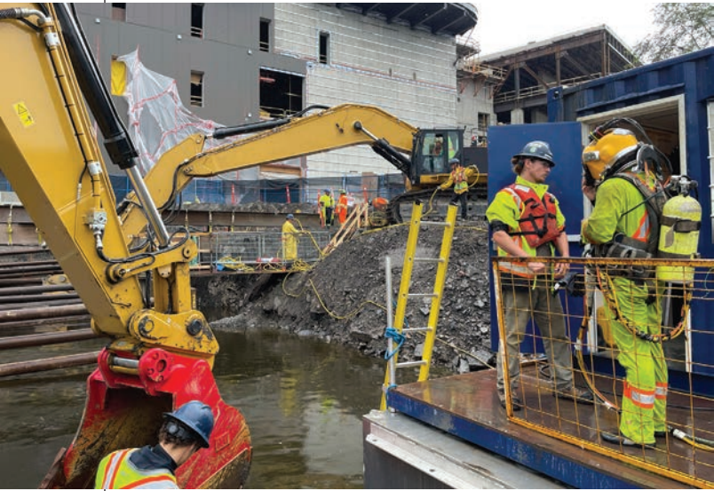
ODS Marine has the capacity to take on projects of any scale, such as the complex ESAP Intake and Outfall Replacement for the City of Ottawa. Photos courtesy of ODS Marine.
