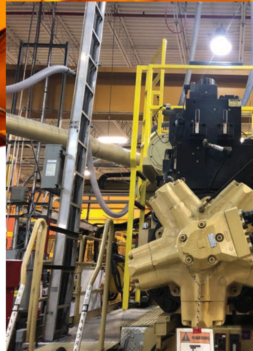
Figure 1: Original Installation. | Installation d'origine.
